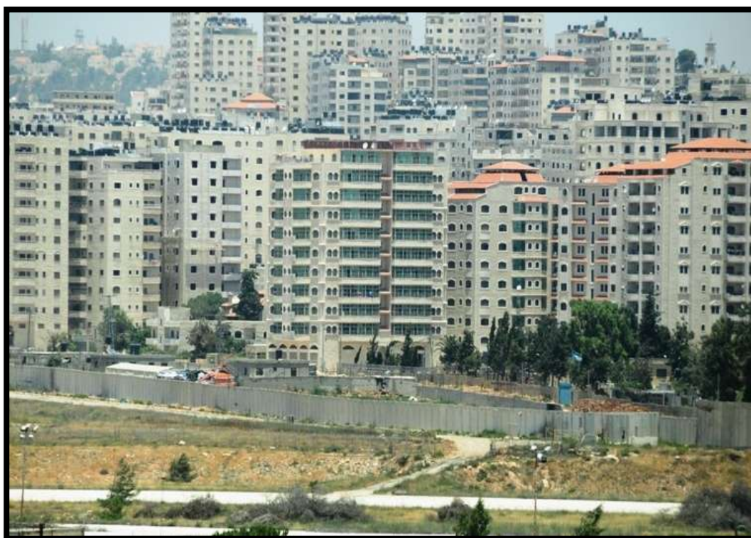
Wild, unsupervised construction beyond the Separation Barrier (SB) in Kafr 'Aqab. Note SB wall. Photo from a tour by Ir Amim and WAC, May, 11, 2014.
